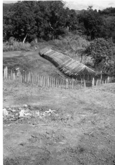
FIGURE 5 General view of the longhouse under completion, showing thatch, roof, and rafters at various stages
