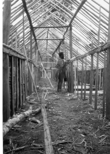
FIGURE 2 Internal view of main central corridor with residence places on either side. The builder is lashing cross-pieces together
