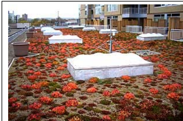
Shadyside Giant Eagle Green Roof (Pop City, 2006).
