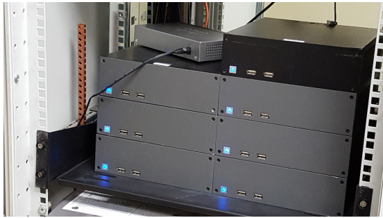
Fig. 6. Close-up of Spire installation shown in Figure 5.
