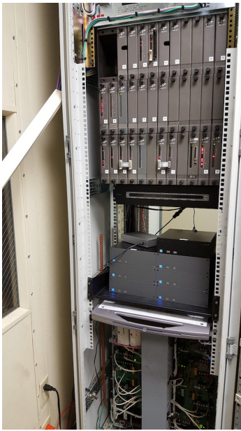
Fig. 5. Spire installed in a DCS room rack at the Hawaiian Electric Company.
